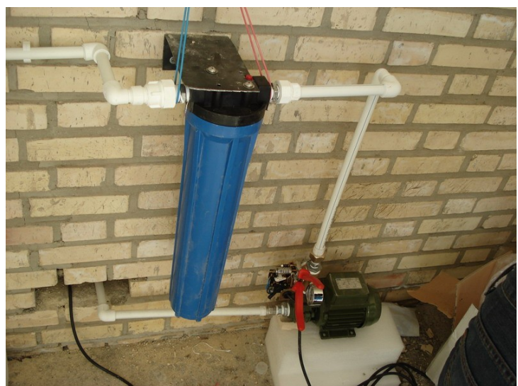
Rust filter prior to ELA-3 000ANW
